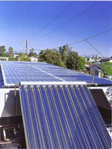
Solar hot-water heaters share rooftop space with PV panels.
